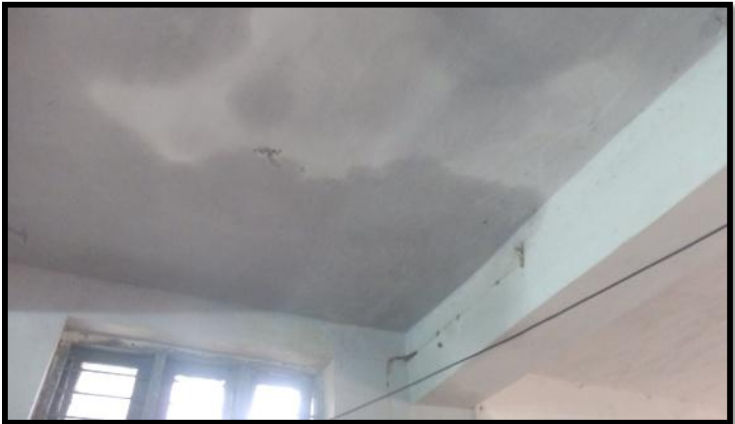
Images showing leakages and withering of slab
