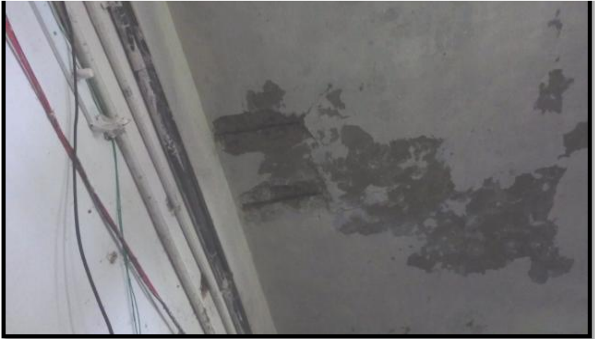
Images showing old electrification ruined.
